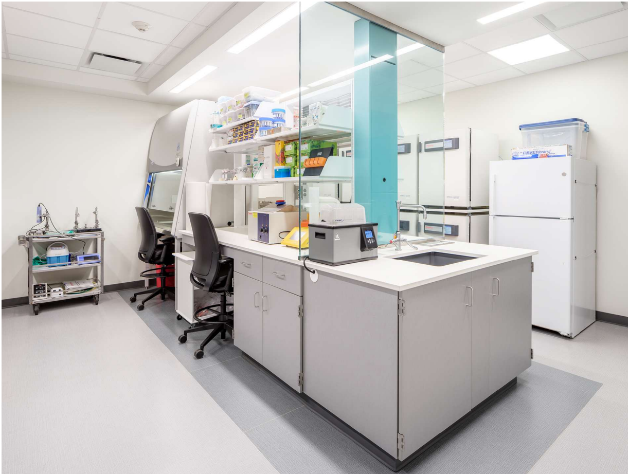
Atrium Health's Cannon Pediatrics Translational Research Lab in Charlotte, NC | Photo Credit: Peter Brentlinger. Product: Max Resistance 2 | Decor: White #0085 CTC | Architect: Little | Installer: New England Lab
